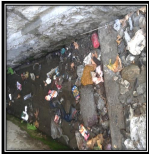
Fig. 2. Human excreta at DHQ hospital MW Filtration Plant.
