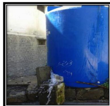
Fig. 1. Fatah Bag WP Leaky overhead water tank.
